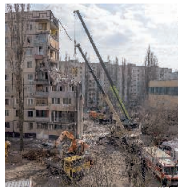
Rescuers clear debris from a multi-story building heavily damaged following a drone strike, in Odesa on Sunday
