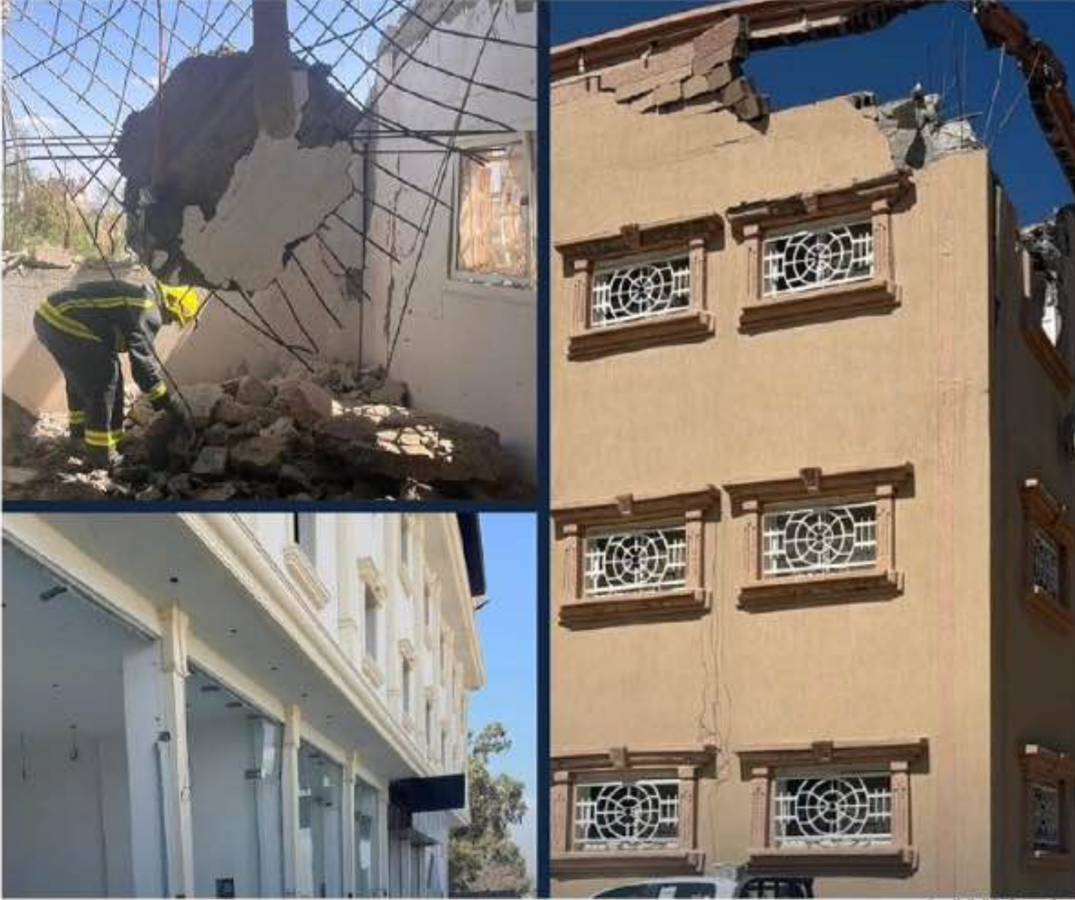
Three residential buildings and seven vehicles sustained damage from the falling debris
