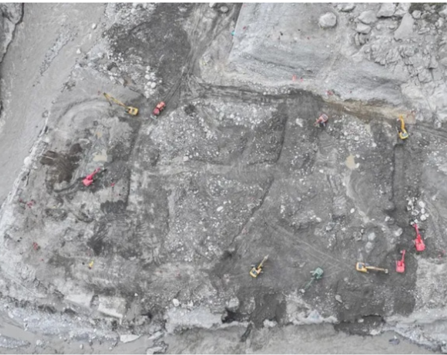
This aerial photo shows excavators working during recovery efforts at the site of the destroyed Gyirong Port border crossing in Gyirong County, in China's western Tibet region on Saturday
