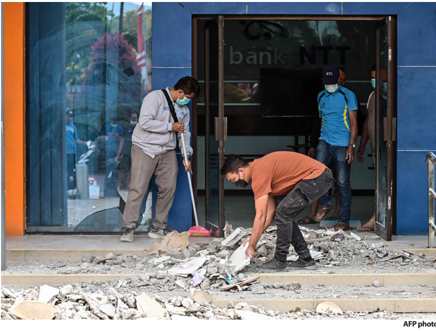
Employees clear debris from a damaged bank building following a 7.7-magnitude earthquake in Ruteng, Manggarai, East Nusa Tenggara, on Sunday
