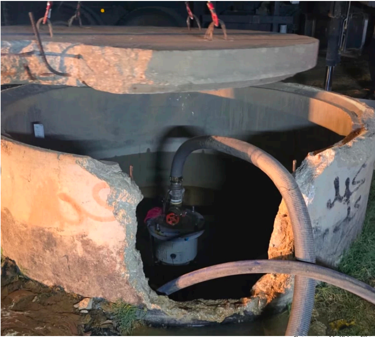
A recent photo of the Ministry of Water and Irrigation shows the latest violation that targeted the Disi Water Conveyance Pipeline in the Jafer area, resulting in the loss of some 5,000 cubic metres of water
