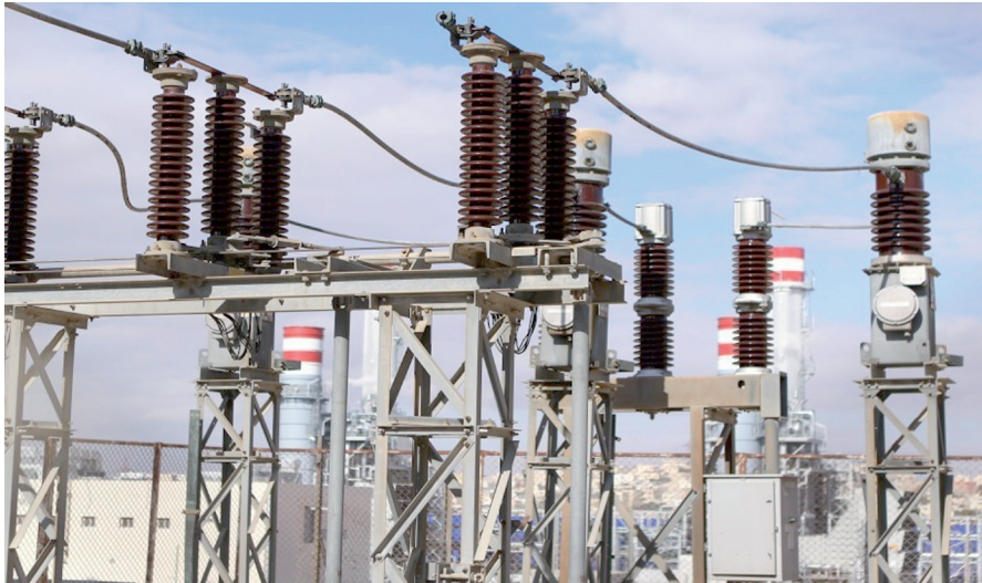
The National Electric Power Company (NEPCO) says that the maximum recorded electricity load on Tuesday reached 4,220 megawatts
