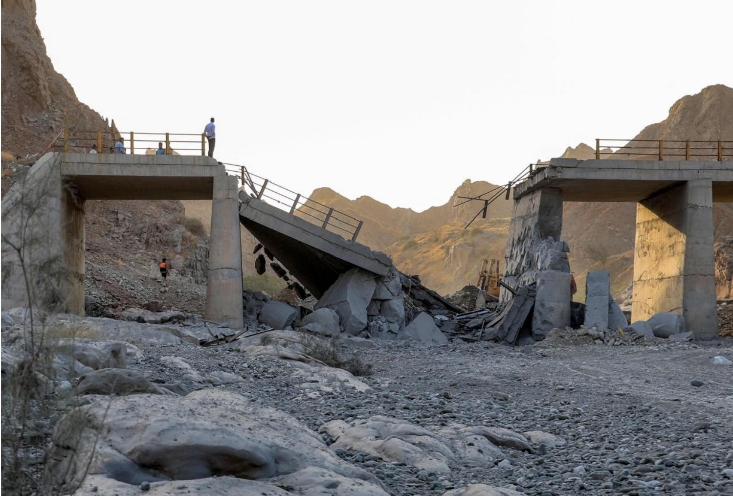
A heavily-damaged bridge which was hit by a US strike is pictured along the road connecting Roudan and Bandar Abbas in southern Iran on Saturday
