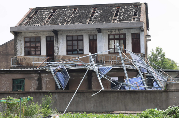
Solar panels damaged by winds from Typhoon Bavi are seen in Wenling, in China's eastern Zhejiang province, on Sunday
