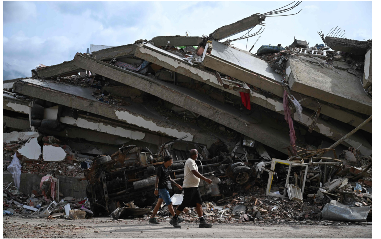
Men walk along the ruins of collapsed buildings in Caraballeda, La Guaira state, Venezuela, on Wednesday, following powerful earthquakes that struck the region
