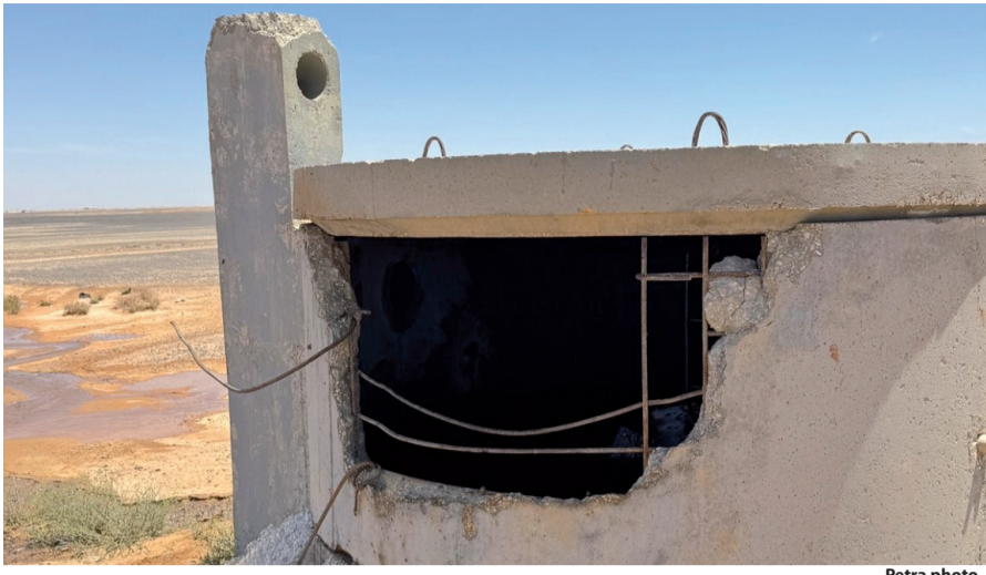
The Ministry of Water and Irrigation and the Water Authority of Jordan detect major violations on the Disi water conveyance pipeline in the Jafr and Manja areas
