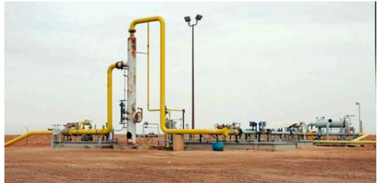
Risha gas field in Ruweished in Mafrqa
