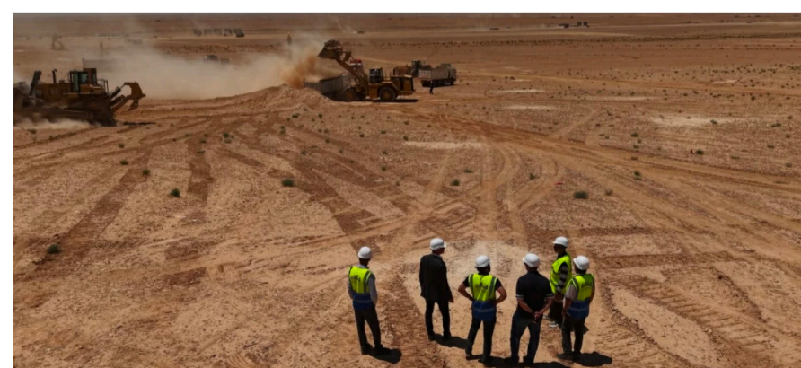
The Jordan Company for the Development of Cities and Facilities announces on Sunday the start of preliminary excavation and site preparation works for the Al Hussein Bin Abdullah II International Stadium project
