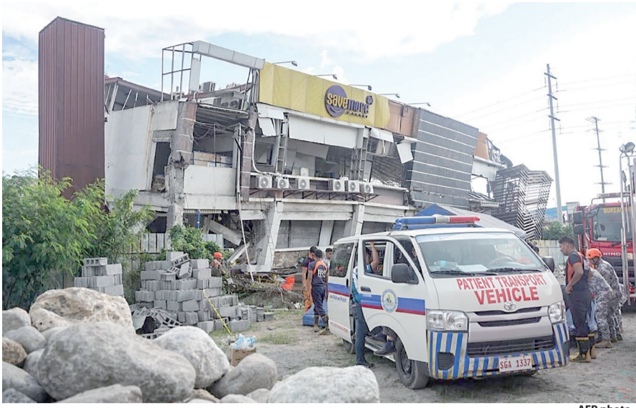
Responders conduct a rescue operation at a collapsed building after a 7.8 magnitude earthquake in General Santos City on Monday
