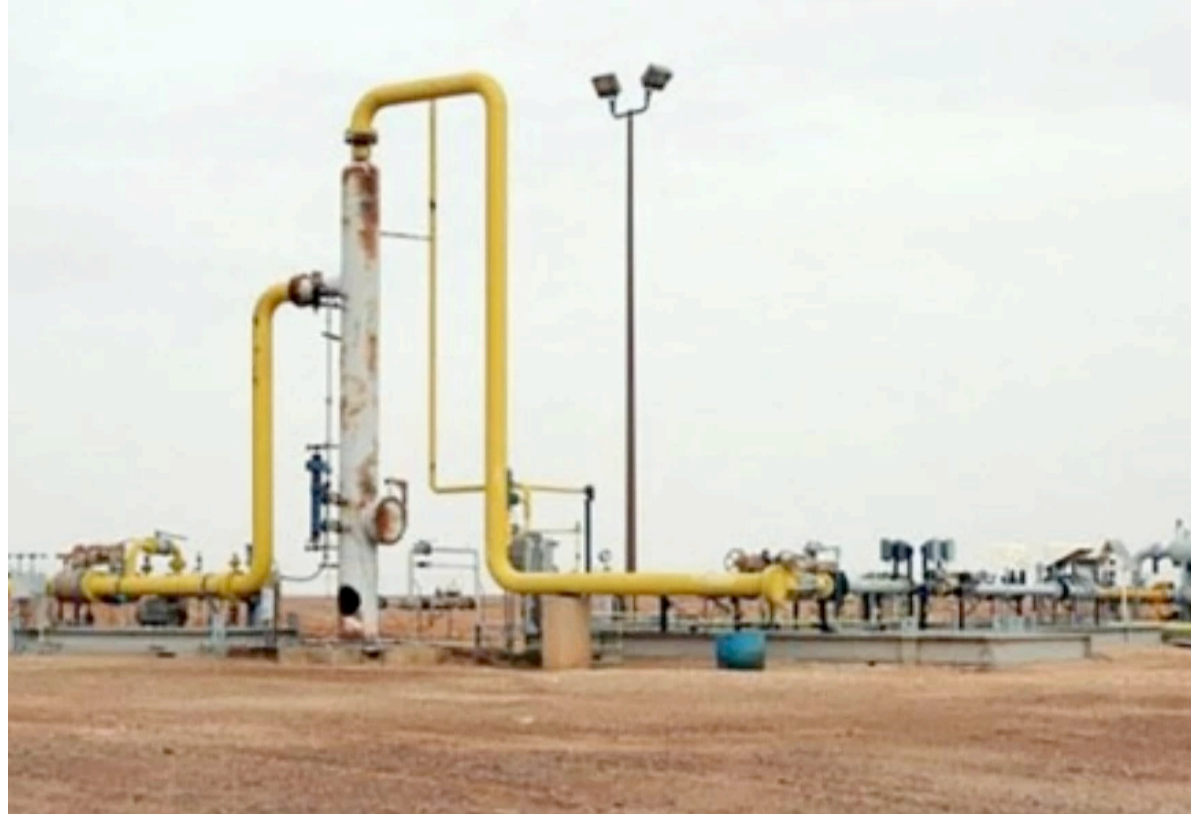
Risha gas field in Ruweished in Mafrqa, some 330 km north of Amman
